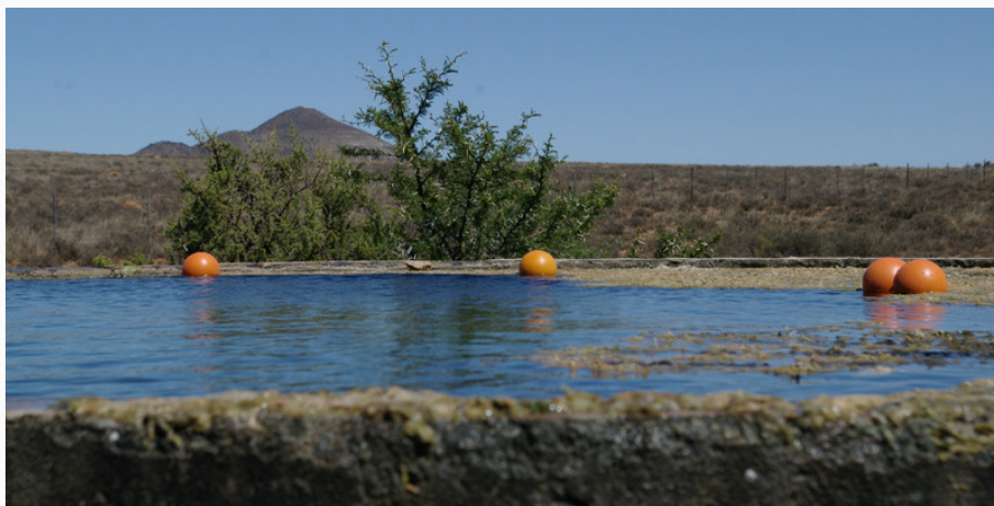
View of reservoir with ballvalves (attachment devices for the suspended unglazed ceramic tiles)
